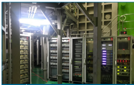
NBI(Neutral Beam Injection) 제어시스템
